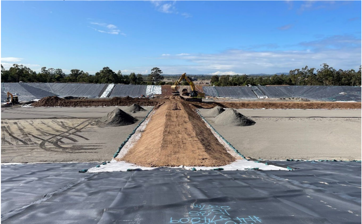
Photo 7: View looking west of construction of internal bunding during Containment Cell construction in April 2022.
