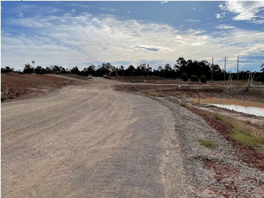
Photo 6: View looking north over Containment Cell temporary access road towards the haul road in May 2022.
