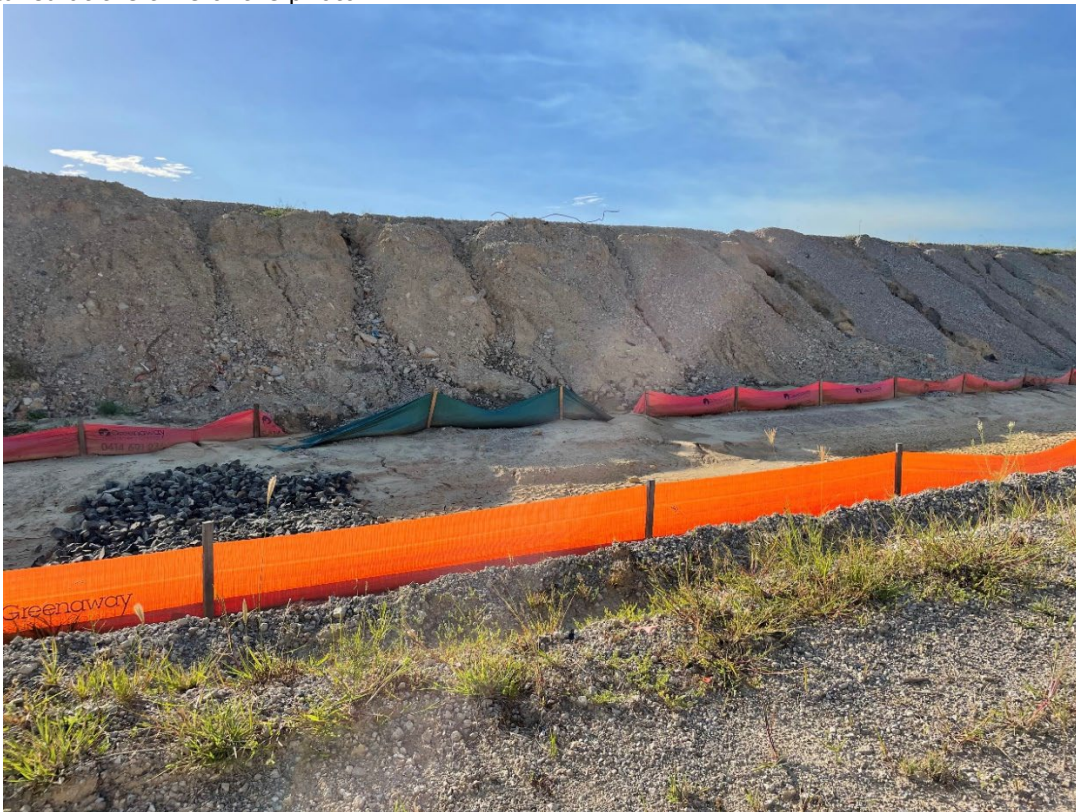
Photo 3: View of clay stockpiles in February 2023. Note the new sediment fencing recently installed at the time of the photo.
