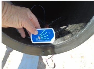
Hydro level sensor installed in the other riser pipe at the south leachate sump (9/2). The sump was emptied on Fri 10/2 in preparation for the start of waste transfer.
