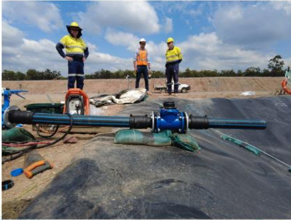
Ready to start commissioning the leachate transfer from the south leachate sump (27/1).
