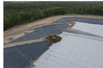
Start of waste transfer to the SE quadrant on Mon 13/2/23. This was the cement-stabilised pond sediments from the west surge pond. An initial pad of 'fluffy' layer material was placed at 1.7m thick using a 36T digger.
