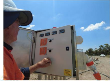
Start/stop control panel for pumping leachate with level indicators for both leachate sumps and both leak detection sumps (25/1).
