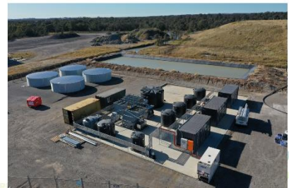
Temporary Water Treatment Plant – final commissioning tests were completed in December. Now undergoing performance testing. Two additional treated water tanks will be installed in February to improve throughput.
