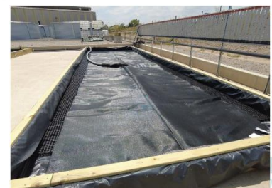
One of two geobags installed at the TWTP for sludge removal (27/1). Trapped sludge and the geobag will be discarded in the ECC.
