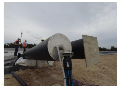
CREA PRO Submersible pump and level sensor installed in the south leachate FUT sump riser pipe (24/1).
