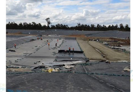
Primary HDPE liner being installed on the floor of the SE quadrant – 11/10/22.
