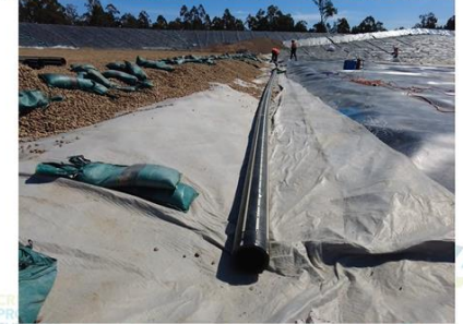
DN160 leachate pipe being installed in drainage trenches of the NW quadrant – 4/10
