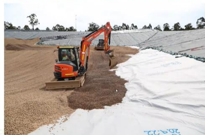
Drainage aggregate deployment in NE quadrant – 21/9/22. Strategic placement using a 6T excavator assists with wrinkle management. Cool wet weather is assisting as liner is more taut.
