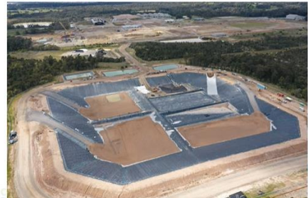
Aerial view of the cell – 18/10/22. A64 geotextile and drainage aggregate installed in three quadrants via the ramps, SE ramp started and work started on south sump.
