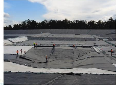
CRG PRO FLU Primary GCL and HDPE being installed in the north sump – 7/9/22
