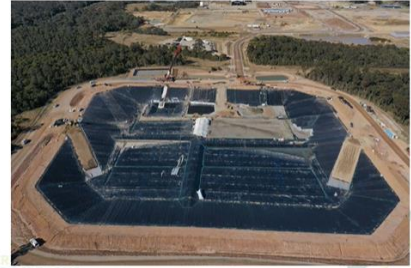
Aerial view of the cell looking east – 18/8/22. Primary liner complete on all batters (except the eastern batter). Primary liner on the floors of the western quadrants are now complete ready for A64 geotextile and drainage aggregate.
