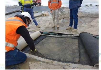
Windows cut into existing liner (HDPE, GCL and GCD) of south sump to inspect the subgrade for damage – 17/10/22.
