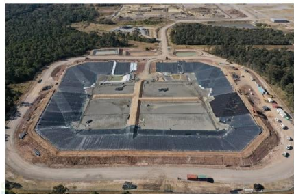
Aerial view of the cell on 16/6/22 showing primary liner (GCD) deployment on the southern batter.
