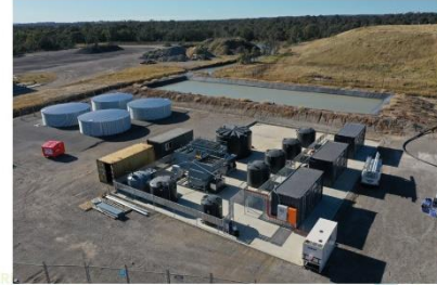
Aerial view of the Temporary Water Treatment Plant on the 16/6/22
